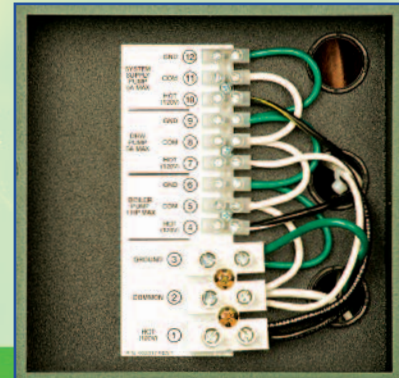
High Voltage Wiring Center (rear of boiler)
