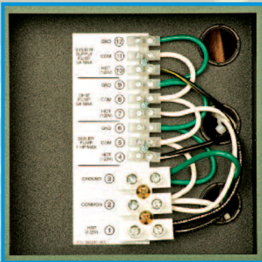
120VAC Wiring Center (rear of boiler)
