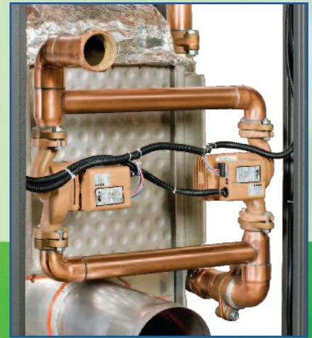
1005A thru 2005A Heating Boiler
